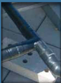
Finished joint ready to withstand the effects of weather and normal wear and tear.
